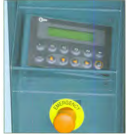
HMI Control Unit
